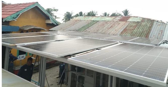
Gambar 3.42 Charging Station Solar Cell
