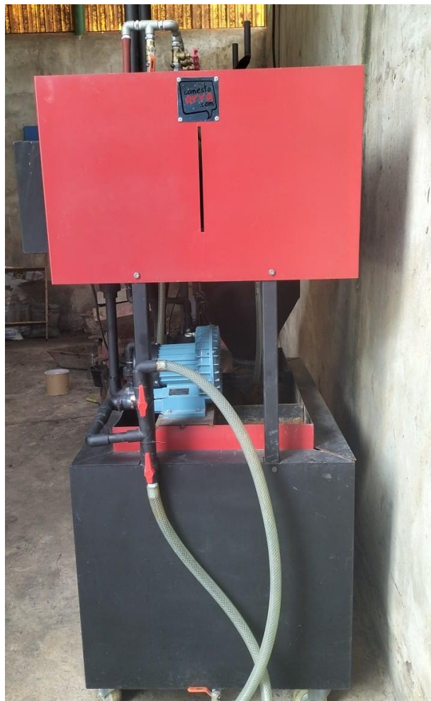
Gambar 3.41 Charging Station Biomassa
