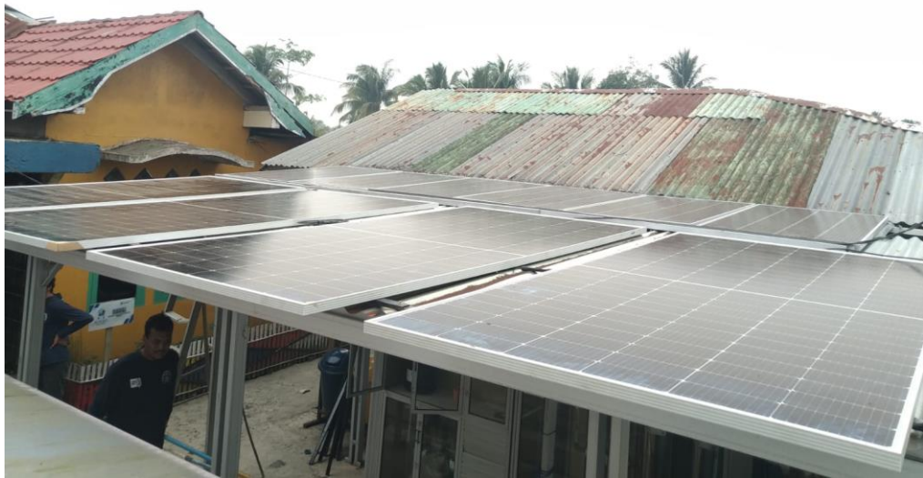
Gambar 5.18 Charging Station Solar Cell
