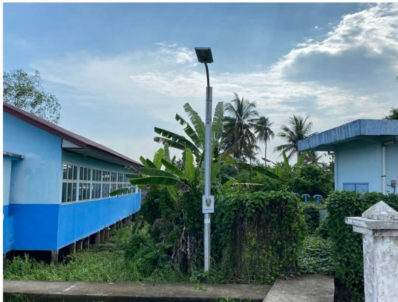
Gambar 5.16 Lampu Penerangan Solar Cell
